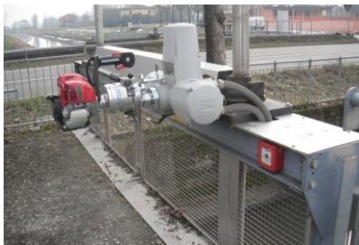
APB/APS tool on BIFFI Electric Actuator
